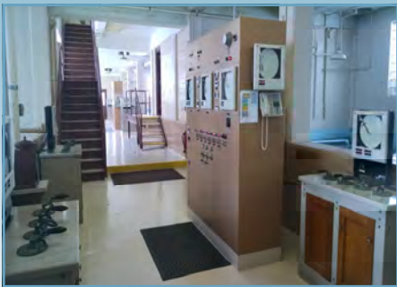
A view of the filter gallery and operations control panel inside the Plant.
