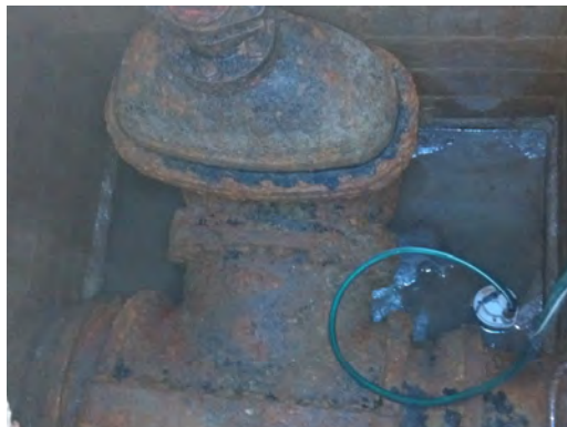
1922 valve needing replacement, located within a concrete vault.
