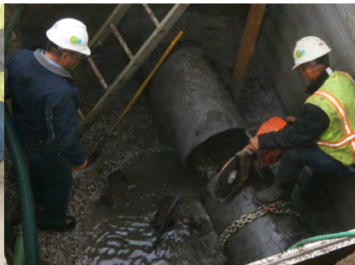
Cutting the pipe outside the valve box, where the new valve and pipe section will be inserted.
